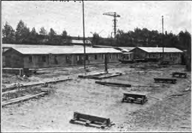
BARRACKS ERECTED BY MEN OF THE U. S. NAVAL RAILWAY BATTERIES. 150-TON CRANE IN THE BACKGROUND.
