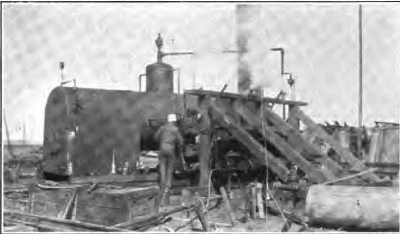
STATIONARY BOILER PUT IN OPERATION AT ST. NAZAIRE FOR FURNISHING POWER FOR COMPRESSED AIR FOR ASSEMBLING THE 14-INCH RAILWAY BATTERIES.
