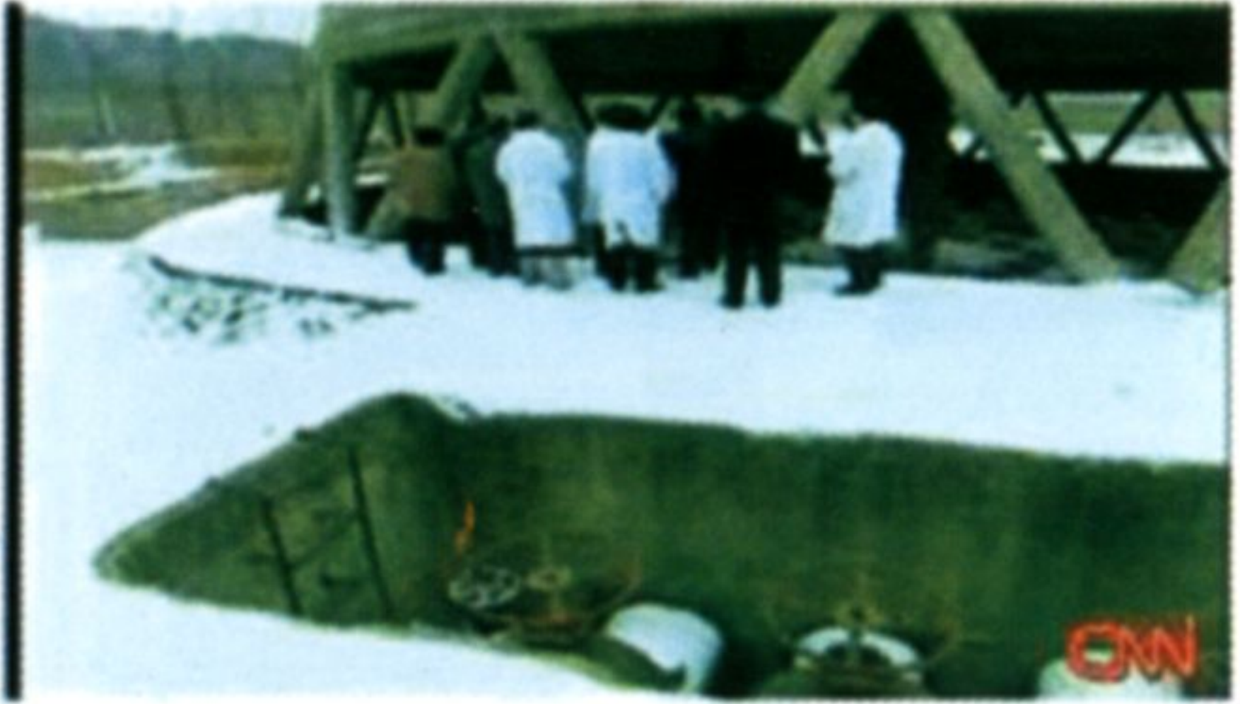
NK Pipes with valve connection between pump house and cooling tower
